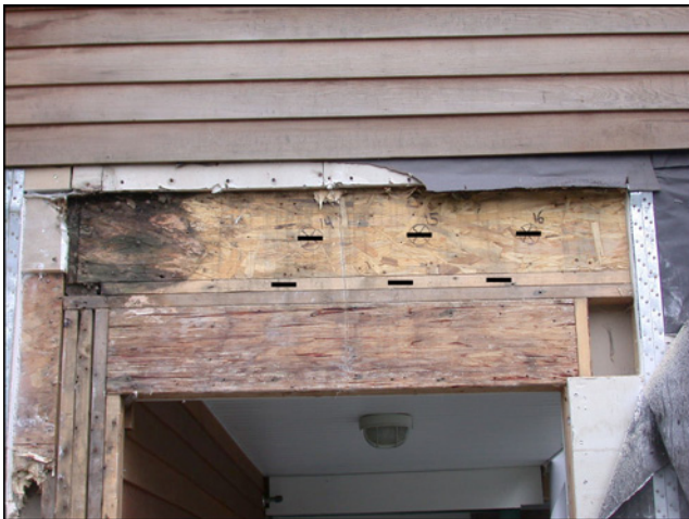
Figure 3—Results at sampling sites in LVL header and door framing under window opening.
