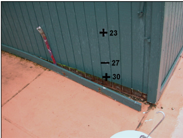
Figure 9—Results at sampling sites in exterior composite siding abutted to poorly drained concrete walkway.
