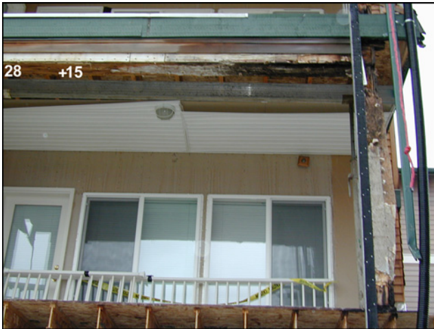
Figure 4—Results at two sampling sites in LVL deck frame.
