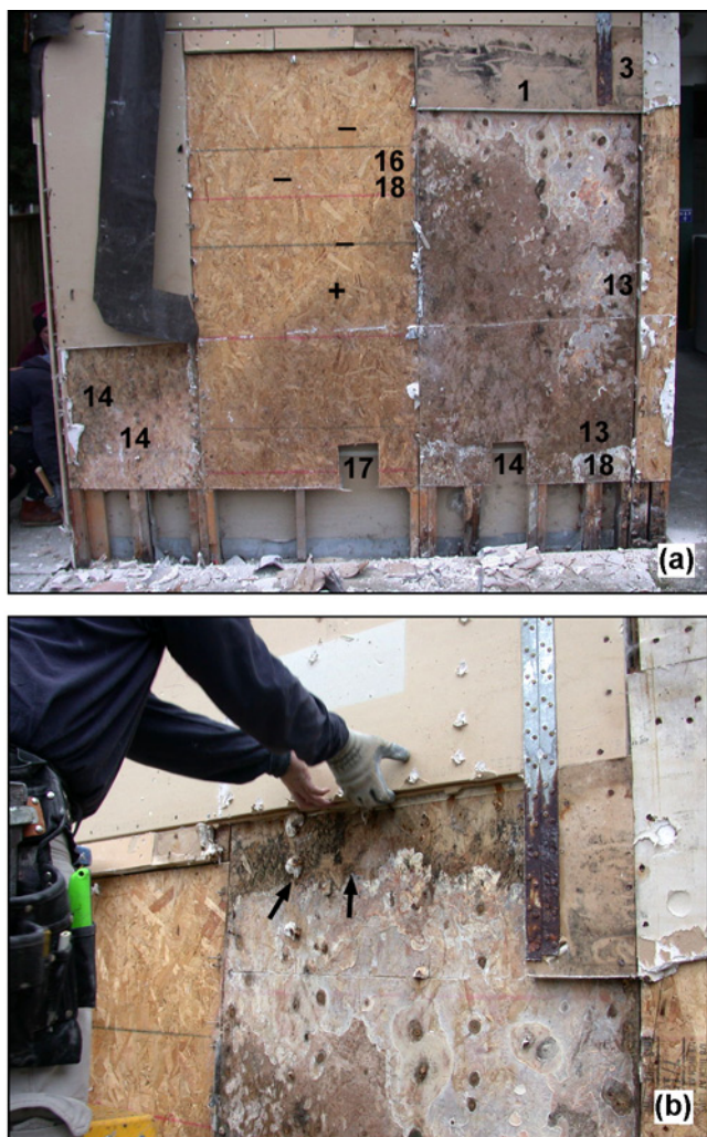
Figure 1—Oriented strandboard (OSB) sheathing beneath window opening. (a) Numerals indicate moisture content (MC) measurements. IWD results recorded as positive (+) or negative (–). (b) Arrows indicate interface between decay and mold fungal growth.
