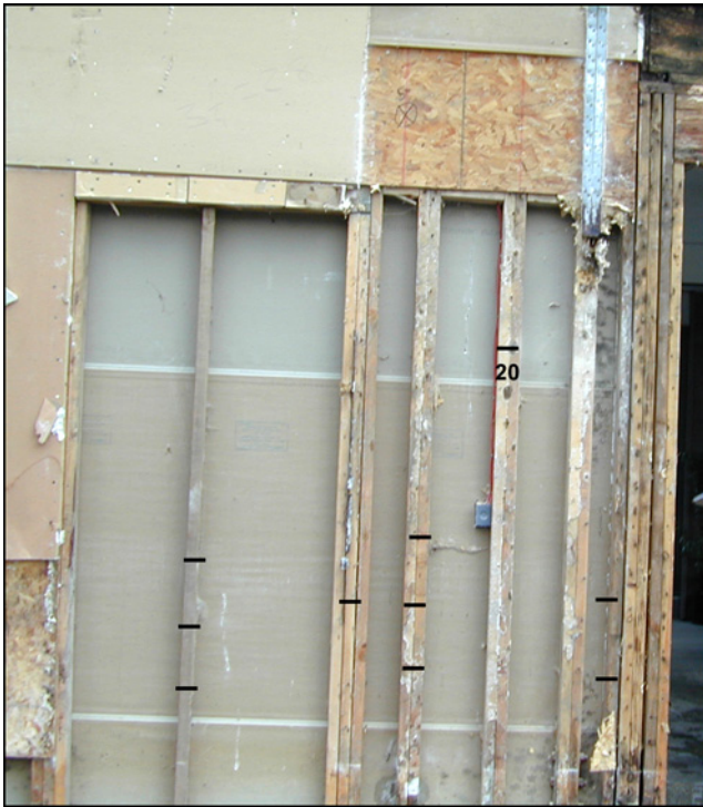
Figure 2—MC measurement (20%) and IWD test results at sampling sites in framing beneath decayed OSB sheathing.
