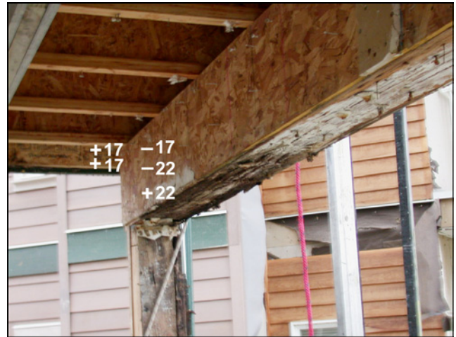
Figure 6—Results at sampling sites in OSB-sheathed deck frame and rim board.
