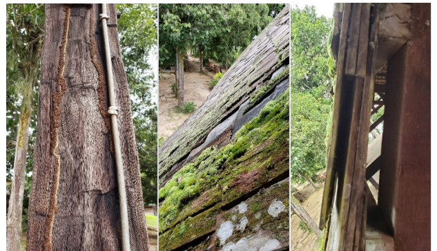
Figure 7— Termites and biodeterioration observed in the timber frame and roof of the Pavilion. Left, arboreal termite damage; center, deteriorated roof shingles, right, delaminated plywood shingles.
