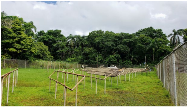
Figure 2— Sherman inland test site. Site has a very high water table and was wet at the time of inspection. It has very little canopy, so it is subject to high UV exposure and more rapid wetting and drying than canopied test sites. Severe decay attack was noted on untreated aspen samples after 6 months.
