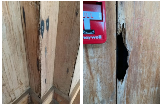
Figure 10—Termite channels, damage, and metal stain spots in the wall inside the cathedral.
