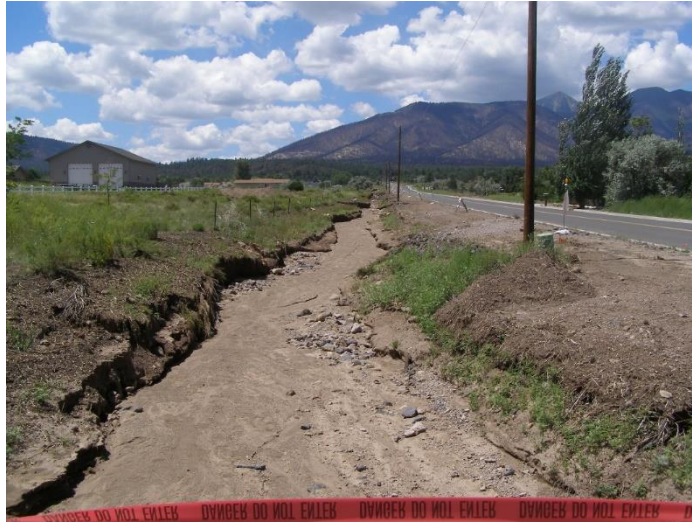
Figure 14. Condition of the Campbell Avenue ditch after the 21 July 2010 storm runoff. Burned runoff source area on the San Francisco Peaks is in the background (Photo by Daniel G. Neary, USDA Forest Service).
