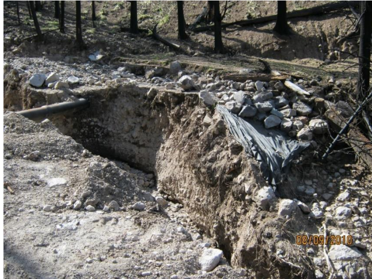
Figure 12. Remnants of a failed structure similar to that shown in Figure 11. The large rocks and boulders, and black plastic sheeting remnants can be seen to the right of the newly incised gully. The gully depth is about 3 m below the original road grade. (Photo by Daniel G. Neary, USDA Forest Service).
