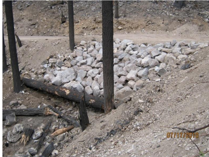
Figure 11. Large rock and boulder rip-rap structure on a road drainage channel immediately after the 2010 Schultz Fire, Coconino National Forest, Arizona, USA (Photo courtesy of Andy Stevenson, Coconino National Forest).
