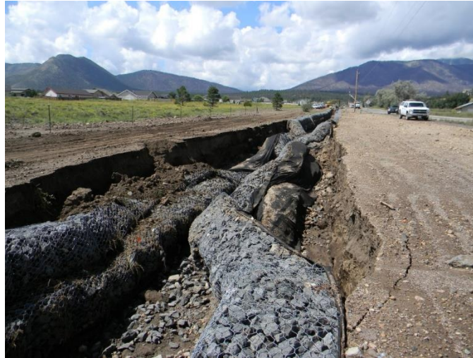
Figure 18. Failure of sections the bank rock-wire gabions in the Campbell Avenue ditch after another storm runoff event. (Photo by Daniel G. Neary, USDA Forest Service).
