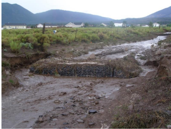
Figure 16. Failure of rock wire gabions in the Campbell Avenue ditch due to design and installation errors after the channel had been upgraded to prevent excessive erosion, 2010 Schultz Fire, Coconino National Forest, Arizona. (Photo by Daniel G. Neary, USDA Forest Service).
