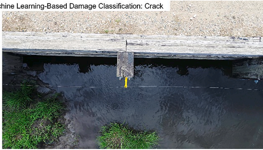
Fig. 12. Representative damage image showing damage classification result.
