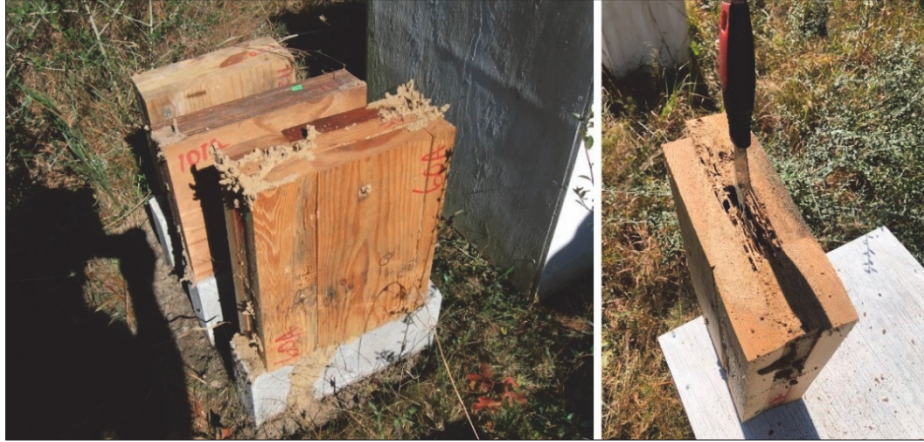
Figure 7. Example of termite attack and damage to 3-ply Douglas-fir CLT in a covered above-ground test after two years.
