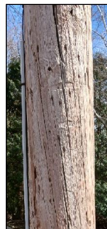
Figure 3— Example of spiral grain in a utility pole.
