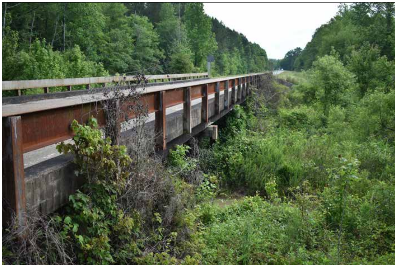
FIGURE 7. Vegetation near to timber bridge elements (Source: Authors). This situation facilitates prolonged moisture exposure and inhibits routine inspection.
