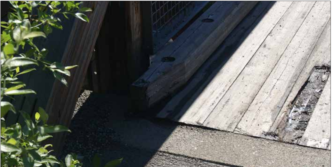
FIGURE 6. Damage on the deck due to water accumulation (Massaro and Malo, 2014).
