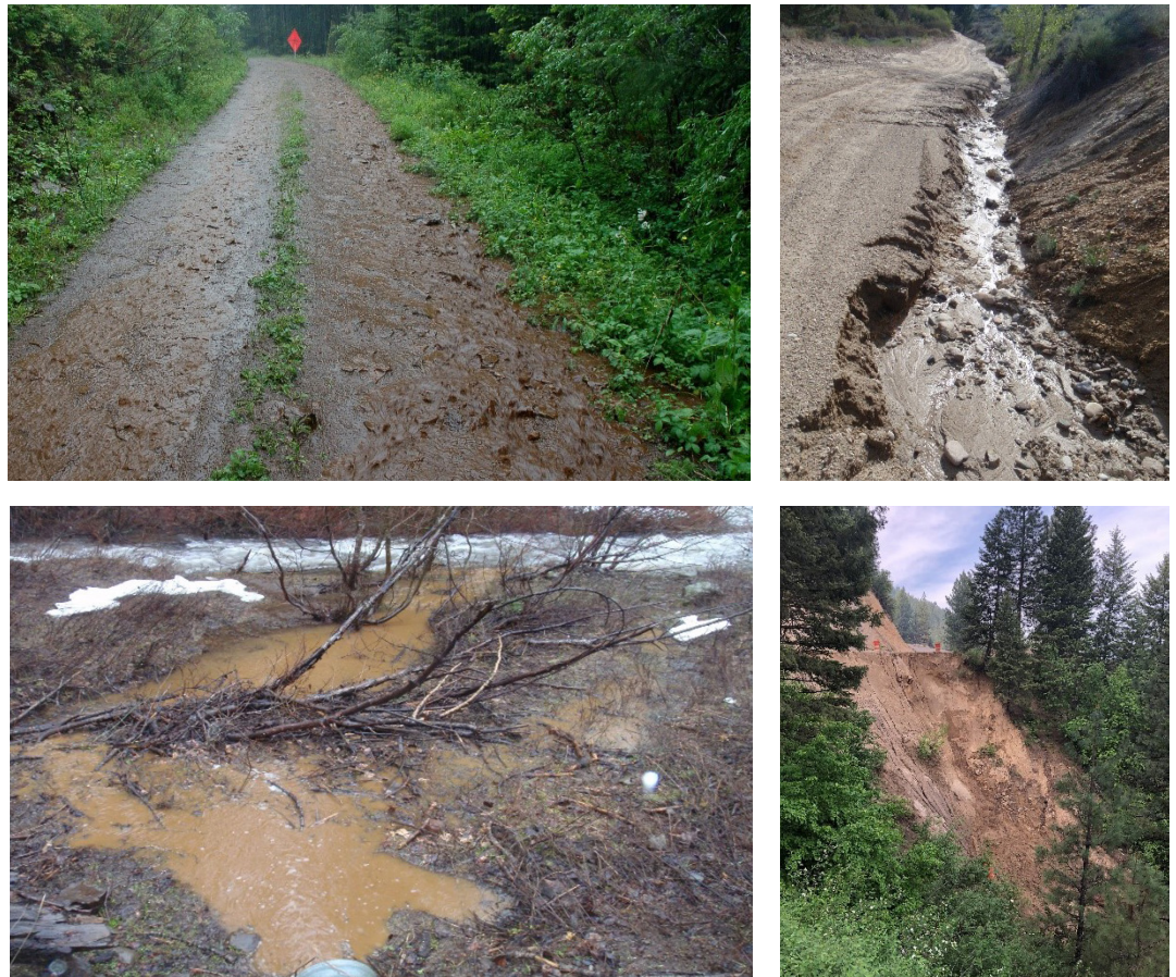
Figure 1: Road surface sediment production, ditch erosion, road fill failure (landslide), and road sediment delivery to a stream. Clockwise from top left.
