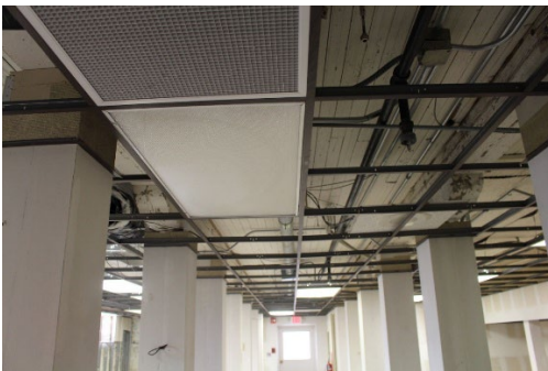
Figure 10—Room 02305. Note horizontal split in timber beam (upper right of photo).
