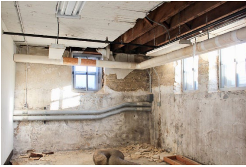
Figure 8—Room 02336, wall damage.
