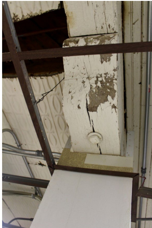
Figure 13—Room 02305. Note horizontal splits surrounding bolt.
