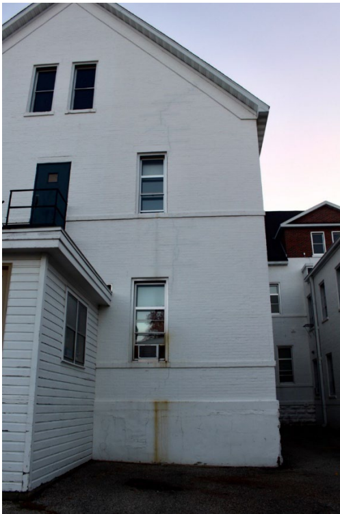
Figure 2—Outside wall. Note crack that extends from the foundation to the roof.
