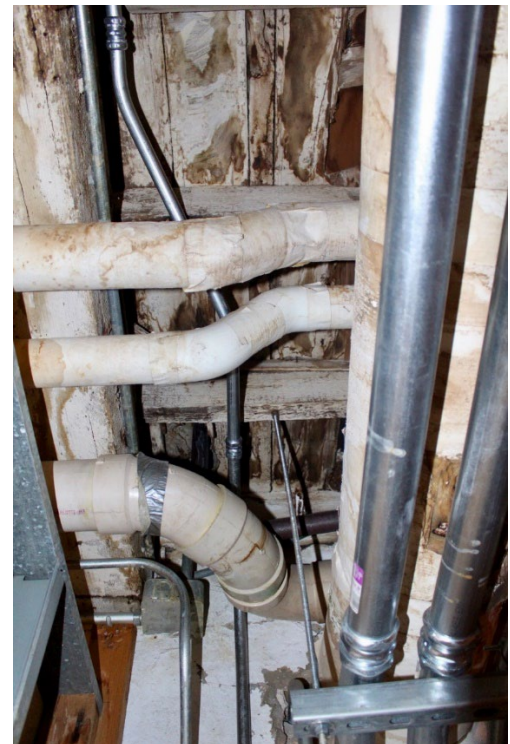
Figure 6—Room 02333, water-damaged floor system.
