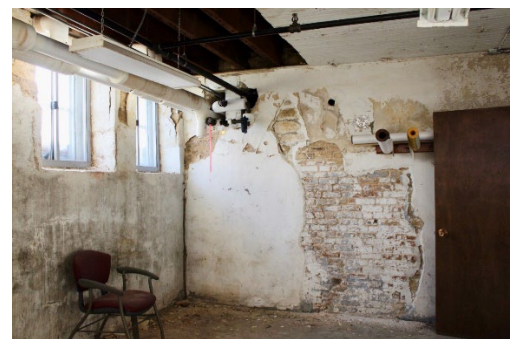
Figure 7—Room 02336, water damage.
