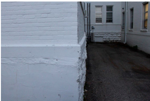
Figure 3—Outside wall. Note outward bowing of the foundation.
