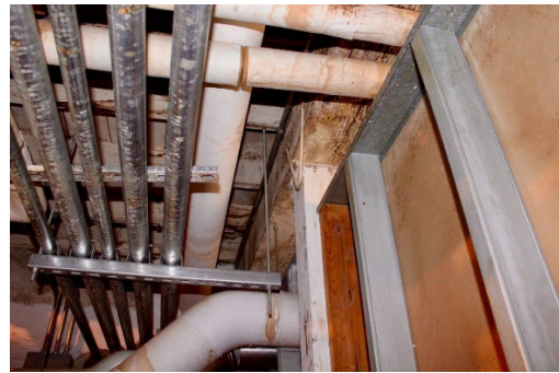
Figure 5—Room 02333, decayed timber beam.
