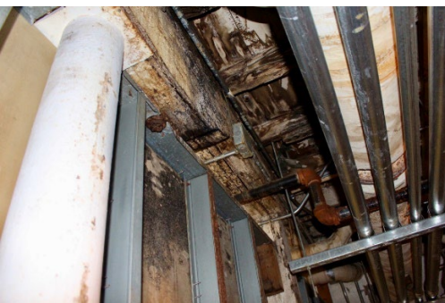
Figure 4—Room 02333, decayed timber beam and water-damaged floor system.
