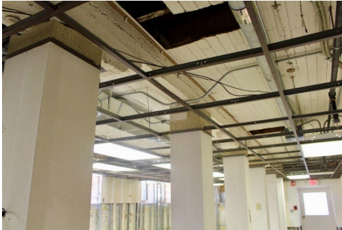
Figure 9—Room 02305. Note horizontal split in timber beam.
