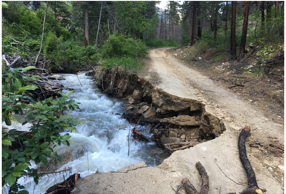
A road paralleling Colson Creek in the Salmon-Challis National Forest is eroding into the channel, disrupting natural channel migration and contributing sediment to the channel. USDA Forest Service photo by Max Smith.
