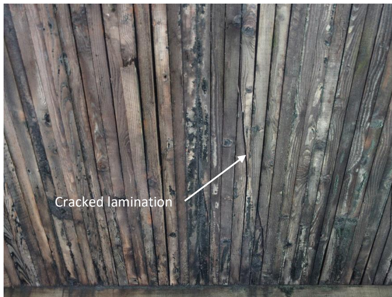
Figure 4-54 Cracked Lamination (La Crosse Co. P320083)
