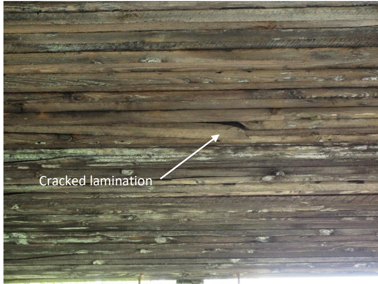
Figure 4-53 Cracked Lamination (La Crosse Co. P320083)
