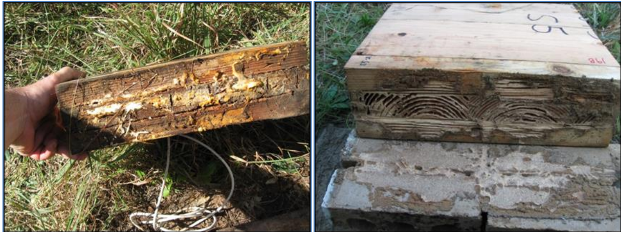
Figure 6: Examples of fungal decay (left) and termite damage (right) to 3-ply Douglas-fir CLT in a covered ground proximity test after six years (picture taken at year 4).
