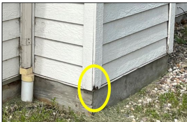
Figure 23—Trim boards around the house are showing signs of decay due to paint failure (photo property of Mississippi State University, used with permission).
