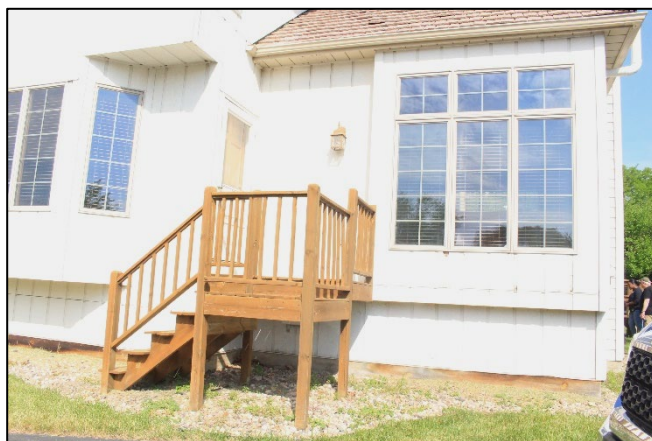
Figure 17—Location of worst siding deterioration beneath and in the vicinity of the triple mullion dining room window (photo property of Mississippi State University, used with permission).
