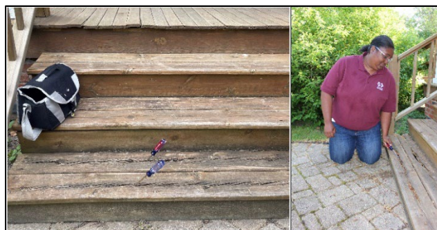
Figure 13 —Screwdrivers were inserted into the decayed portions of the steps to the front porch, showing the extent of the deterioration (photos property of Mississippi State University, used with permission).
