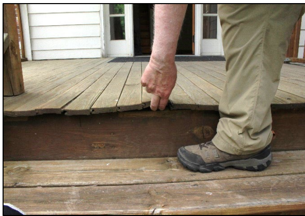
Figure 14—The front porch flooring near the top of the steps has become unfastened due to fastener corrosion (photo property of Mississippi State University, used with permission).
