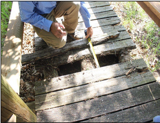
Figure 7—Deteriorated deck boards in the accessibility ramp. Some of the deck boards could be removed without effort (photo property of Mississippi State University, used with permission).
