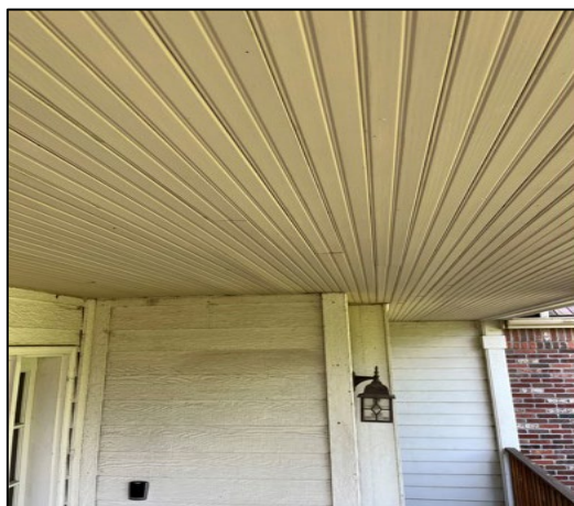
Figure 16—Tongue and groove ceiling of the front porch is swelling, indicating moisture issues (photo property of Mississippi State University, used with permission).
