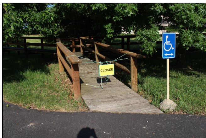
Figure 10 —“Closed” sign and rope barricade at one of three entrance points to the accessibility ramp (photo property of Mississippi State University, used with permission).
