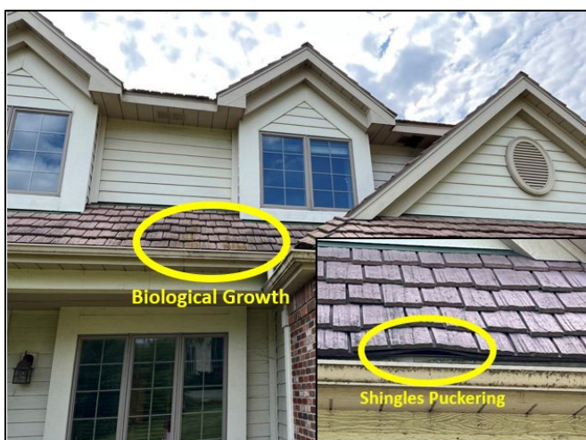
Figure 24—Shingles showing signs of weathering, such as biological growth and puckering (photo property of Mississippi State University, used with permission).
