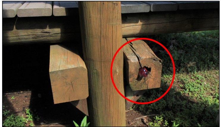
Figure 9—Advanced decay in carrying beams that support the floor frame of the accessibility ramp (photo property of Mississippi State University, used with permission).
