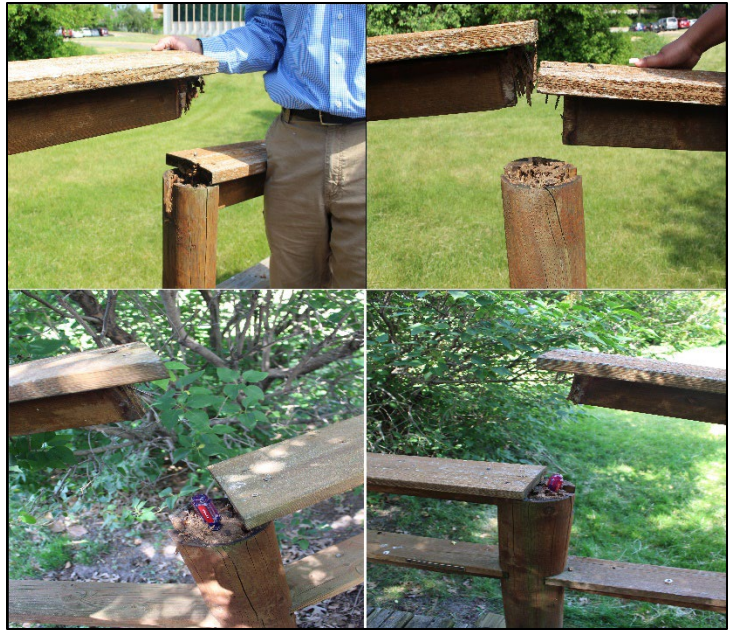
Figure 8—Rail-to-post connections in the accessibility ramp were severely decayed. The rail can be removed from the post, and the post was also decayed. When the post was probed with a screwdriver, the screwdriver went in easily (photos property of Mississippi State University, used with permission).
