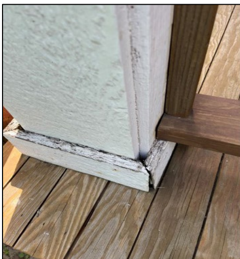
Figure 15—Front porch post trim showing signs of deterioration (photo property of Mississippi State University, used with permission).
