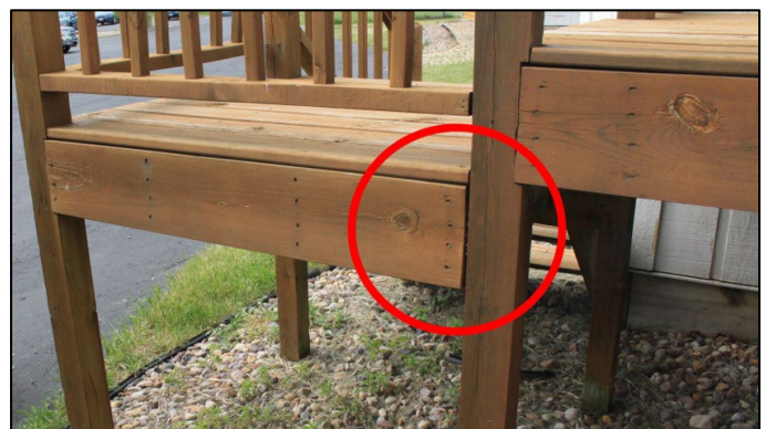
Figure 3—Joist-box-to-rail connection of back entrance deck showing insufficient fixity (photo property of Mississippi State University, used with permission).
