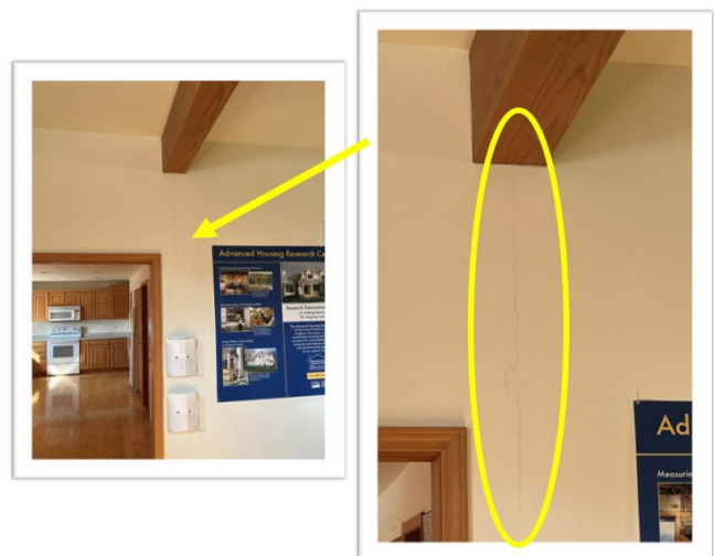
Figure 25—A fracture or buckling of sheet rock in the great room. The right-side header inside the great room shows fracture or buckling in the drywall above the door opening. This may correspond to soil settling or foundation movement on the left side in the basement (photos property of Mississippi State University, used with permission).
