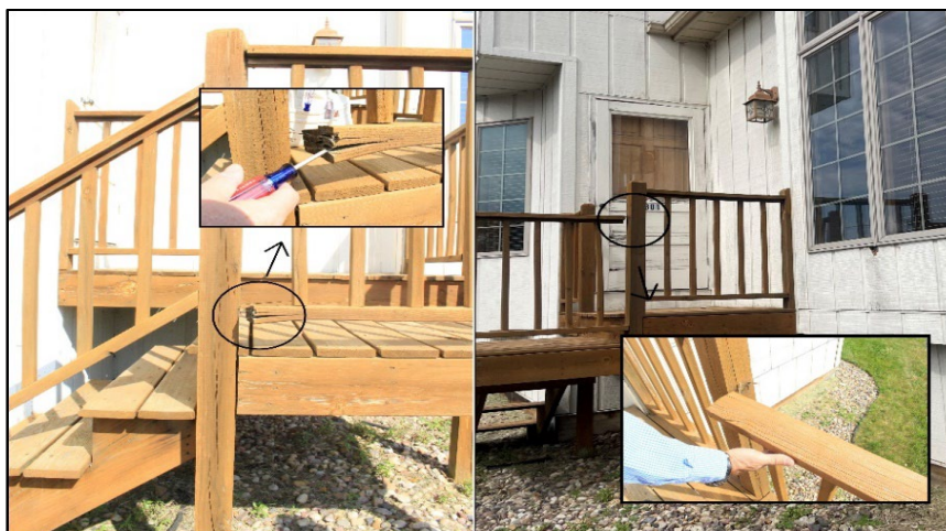
Figure 5—Rail-to-post connections of the back entrance have completely failed in the highlighted locations (photos property of Mississippi State University, used with permission).
