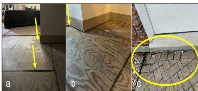
Figure 26—Signs of settling in the foundation in the southwest portion of the basement (a and b) and in front of the garage (c). The treated plywood foundation shows unleveling underneath the left side pier supporting the left side great room wall (a and b). This may have been caused by water movement under the foundation. Other indications of water can be seen in the soil unleveling under the pavers located near the front left side of the garage approach (c) (photos property of Mississippi State University, used with permission).
