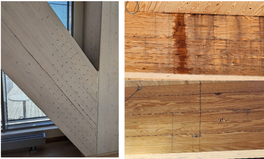
Fig. 1. Cracks in glue-laminated timber elements: diagonal brace (left) and beams supporting CLT floor panels (right).
