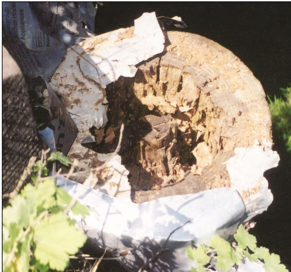
Figure 1.11—Damage to a bridge piling.
