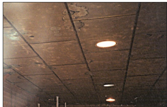
Figure 1.6—The ceiling panels were stained and discolored.
