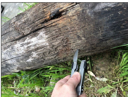
Figure 7.10 —The knife blade is driven approximately 3/8 in. into the shell of a utility pole.
