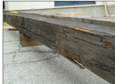
Surface decay and multiple cracks
