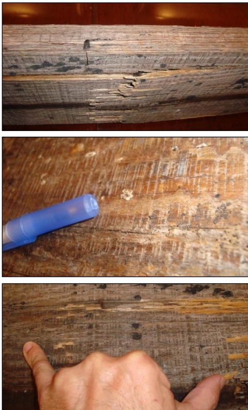
Figure 7.2—Fractured piece of laminated veneer lumber scaffold planking. Before use, cursory observation suggested that the specimen was sound. However, examination after fracture noted multiple fungal fruiting bodies, indicating advanced decay, in relatively close proximity to the fracture. Ballpoint pen cap and hand indicate the size of fungal fruiting body and its proximity to the fracture, respectively.
