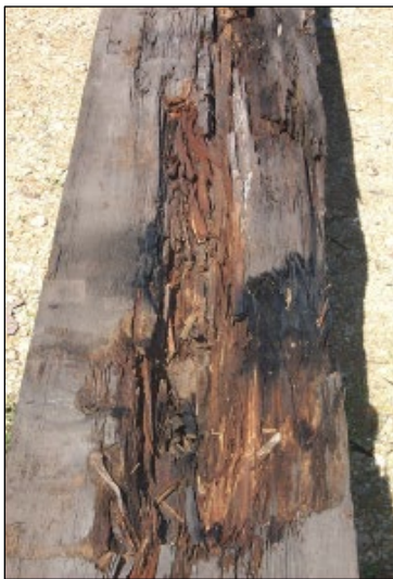
Severe decay damage
