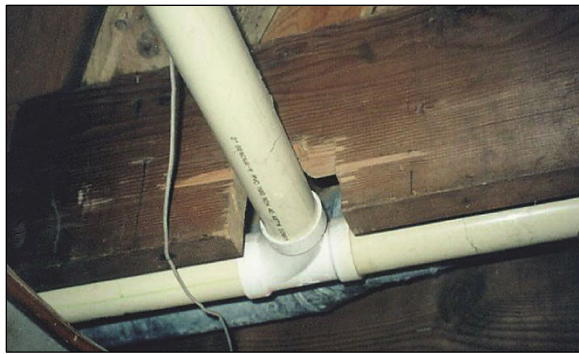
Figure 1.16—A floor joist was cut to make room for plumbing. This should never be done.
