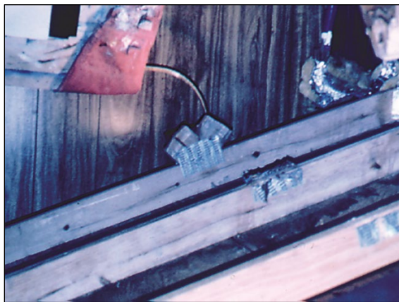
Figure 1.13—Metal plate connectors were cut and bent so that the webs could be removed. This should never be done.
