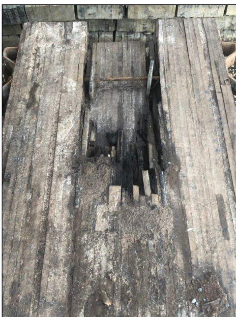
Figure 7.1—Wood mat composed of three pressure-treated glued-laminated timbers with a broken middle member. This mat can be disassembled, repaired, and returned to service.
