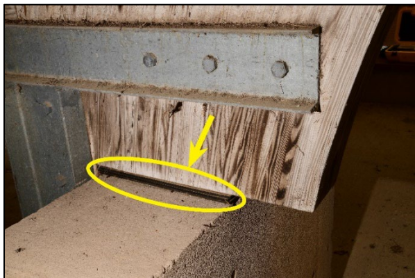
Figure 8—Barrier material designed to prevent moisture transfer from concrete to glulam supports.
