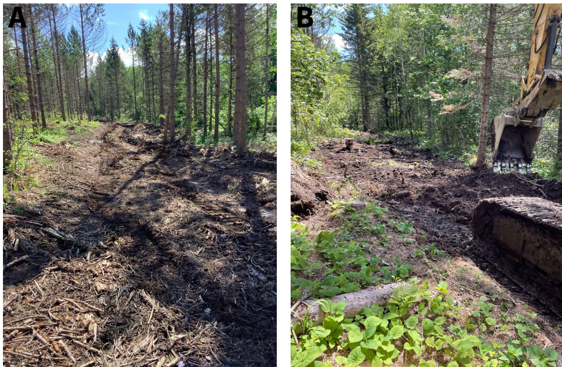
Figure 11. —Skid trail (A) before and (B) during and after remediation for rutting and compaction. USDA Forest Service photos.
