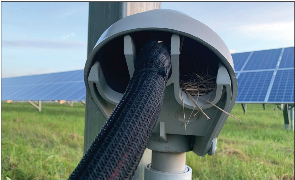
Figure 3. Eastern Bluebird nest placement inside of the weather hood for electrical cables at a PV solar energy facility, 1 July 2022, Albany County, NY.
