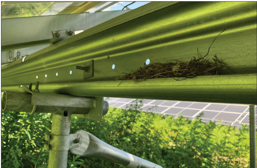
Figure 1. Eastern Bluebird nest on the bottom steel shelf of the racking structure supporting photovoltaic (PV) solar panel modules at a PV solar energy facility, 17 June 2022, Ulster County, NY.
