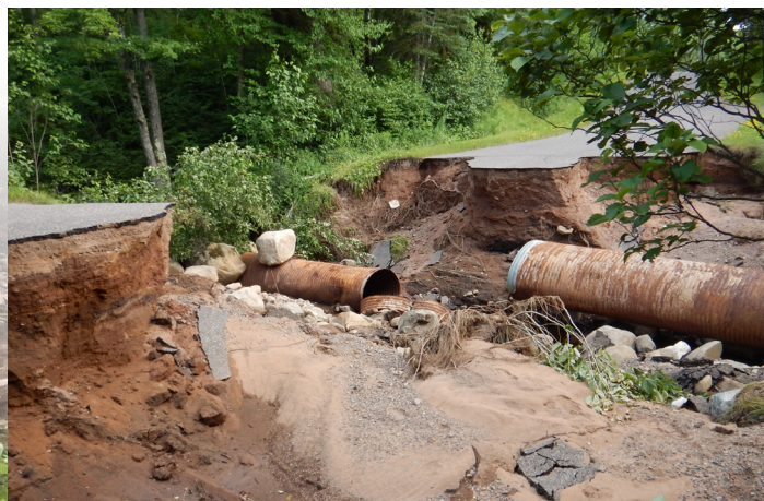
A failed traditional crossing at the Chequamegon-Nicolet National Forest following the 2016 flood. USDA Forest Service photo by Dale Higgins.
