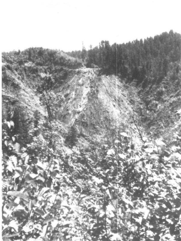
Figure 24.--Land overhang. It is not uncommon for landings to be constructed in such a manner as to have sidecast material form very steep slopes. This is a poor construction practice. This problem is often compounded by piling cull material on the edge. The edge of the landing can fail causing damage on and off site.
