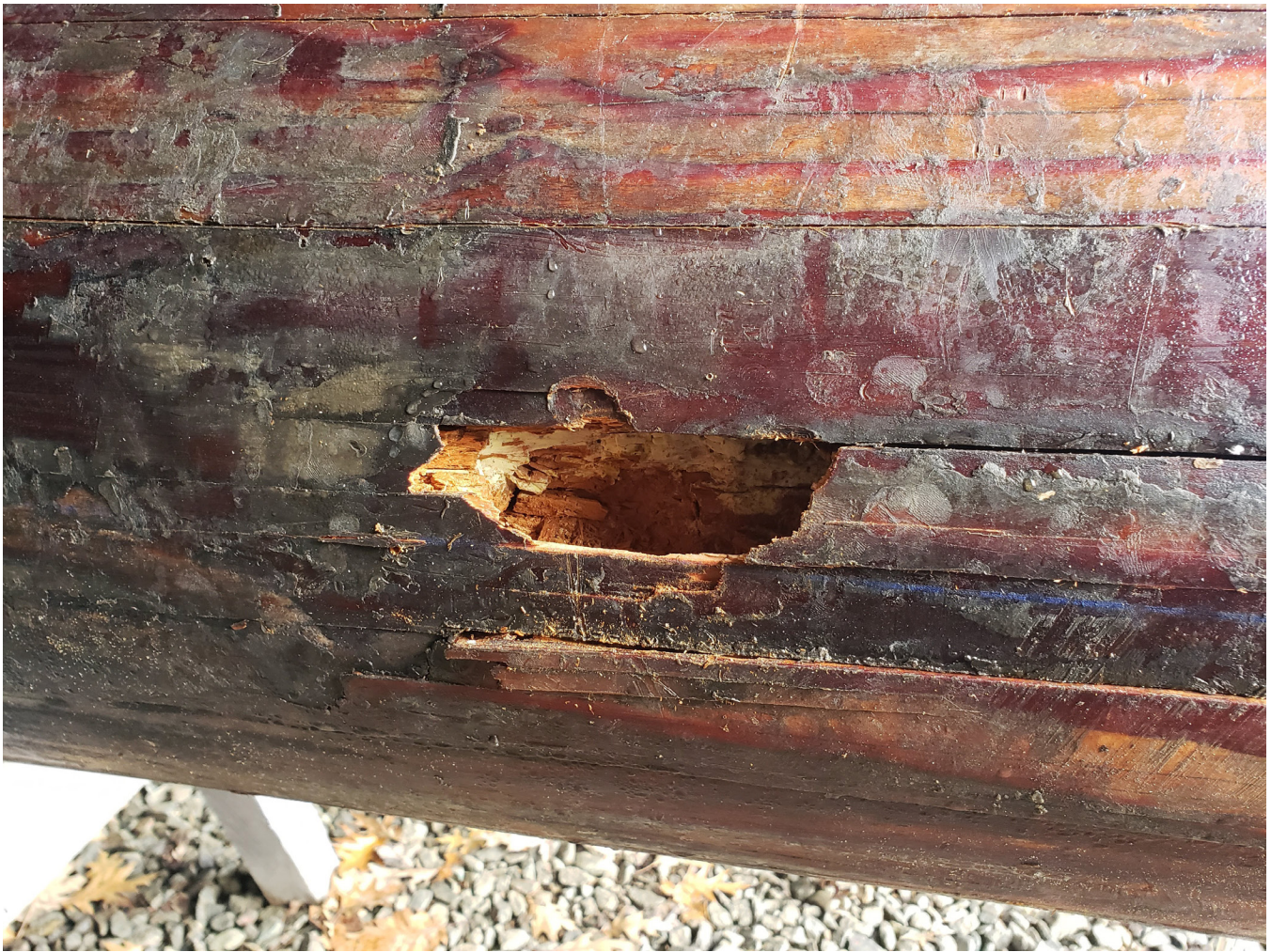
Figure 1G. —Examination hole in the Grace Bailey mast (at approximately 39 ft) created prior to Forest Products Laboratory inspection and revealing internal decay. Forest Service photo by Xiping Wang.
