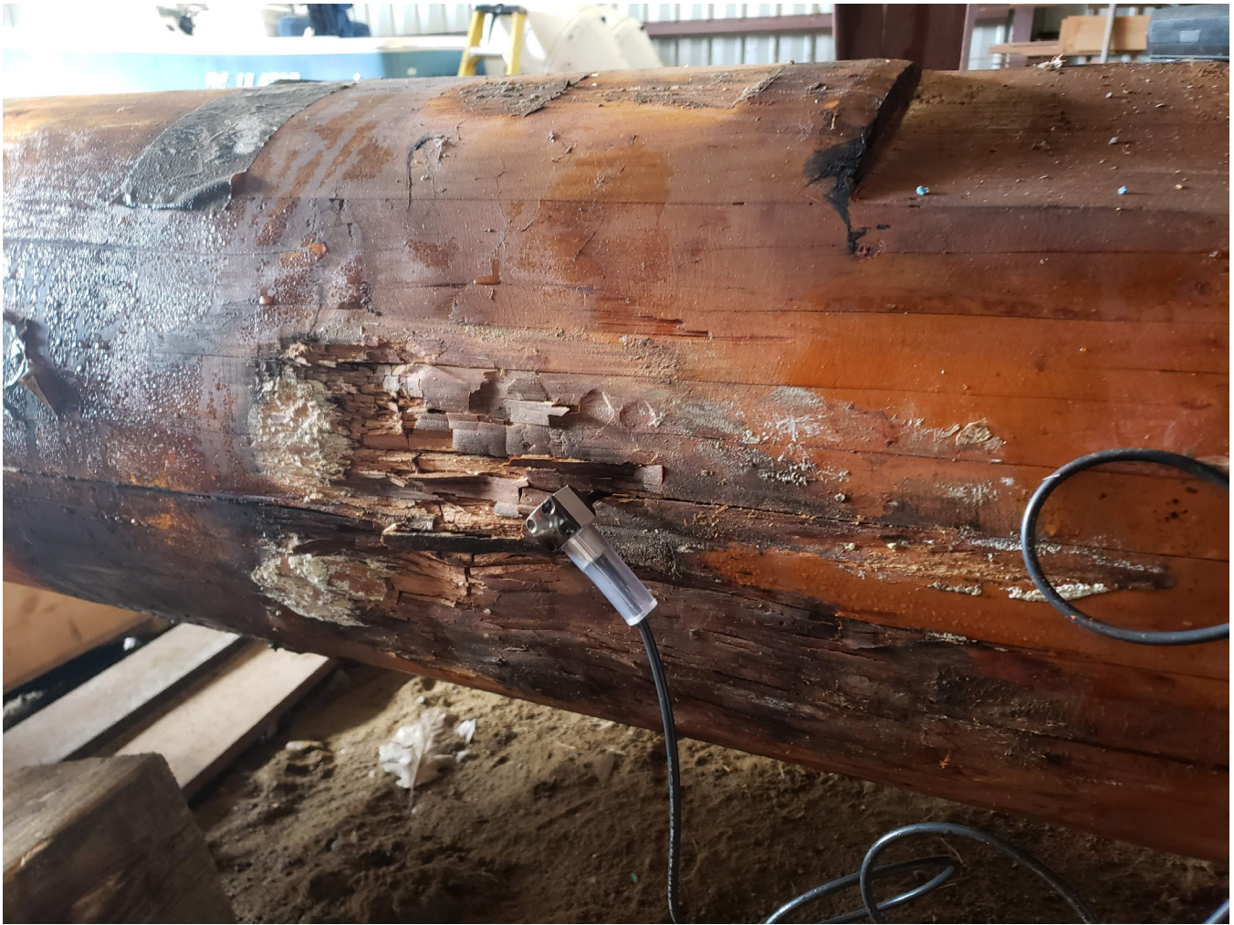
Figure 1L. —Surface deterioration observed on the Grace Bailey mast at 5 ft. Forest Service photo by Xiping Wang.
