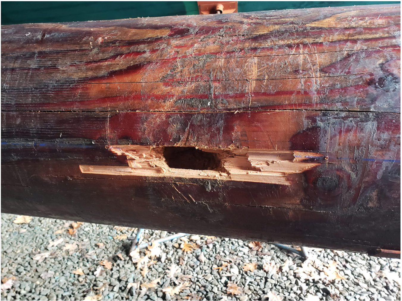
Figure 1H. —Examination hole in the Grace Bailey mast (at approximately 34 ft) created prior to Forest Products Laboratory inspection and revealing internal decay. Forest Service photo by Xiping Wang.
