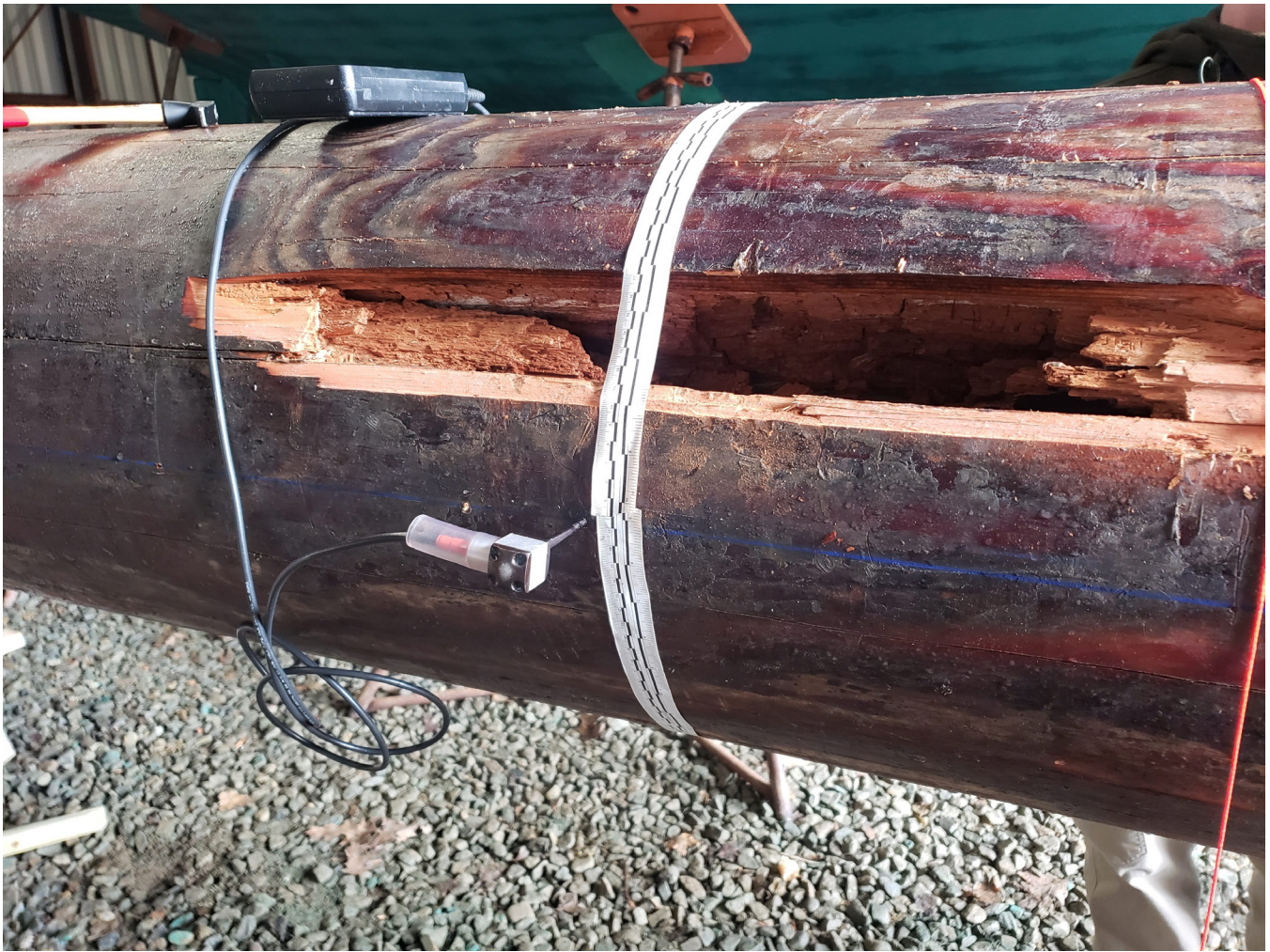
Figure 11. —Opening in the Grace Bailey mast (at approximately 25 ft) created prior to Forest Products Laboratory inspection and revealing internal decay. Forest Service photo by Xiping Wang.
