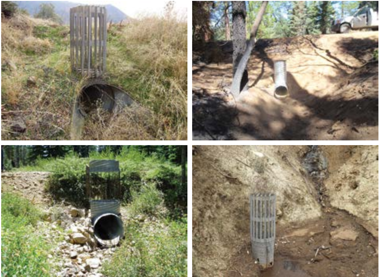
Figure 4.42—Culverts with plugging potential (top) and trash racks to prevent plugging (bottom) that have been designed with different trash rack risers in areas where wildfire has occurred. Upper photos by Joshua Direen, USDA Forest Service, San Bernardino National Forest; lower photos by Gordon Keller.
