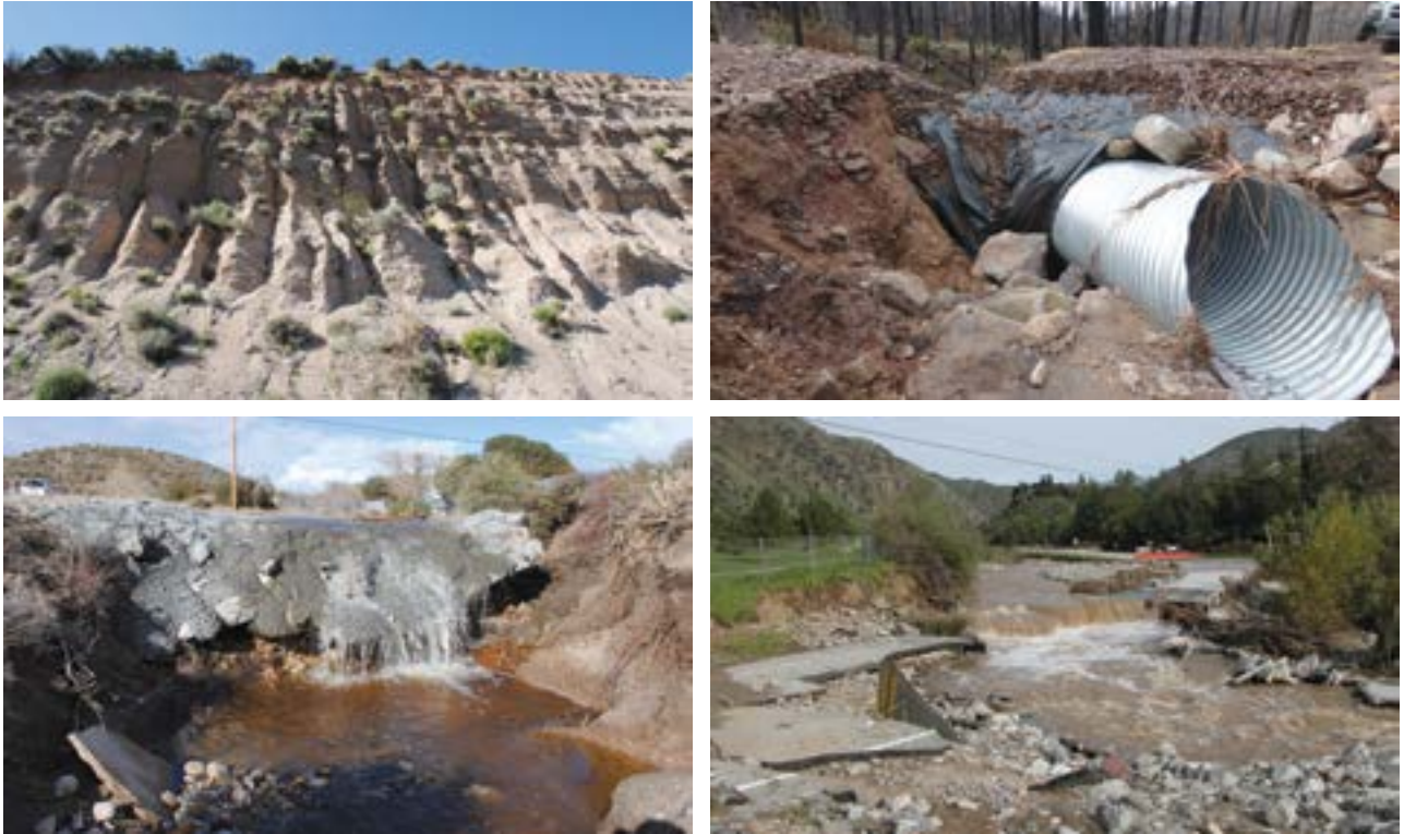
Figure 4.3—Examples of southern California forest roads with erosion and infrastructure, including culverts and fords damaged by flooding, storms, and fires. Left photos by Vincent Barandino, USDA Forest Service, National Technology and Development Program; right photos by Donald Lindsay.
