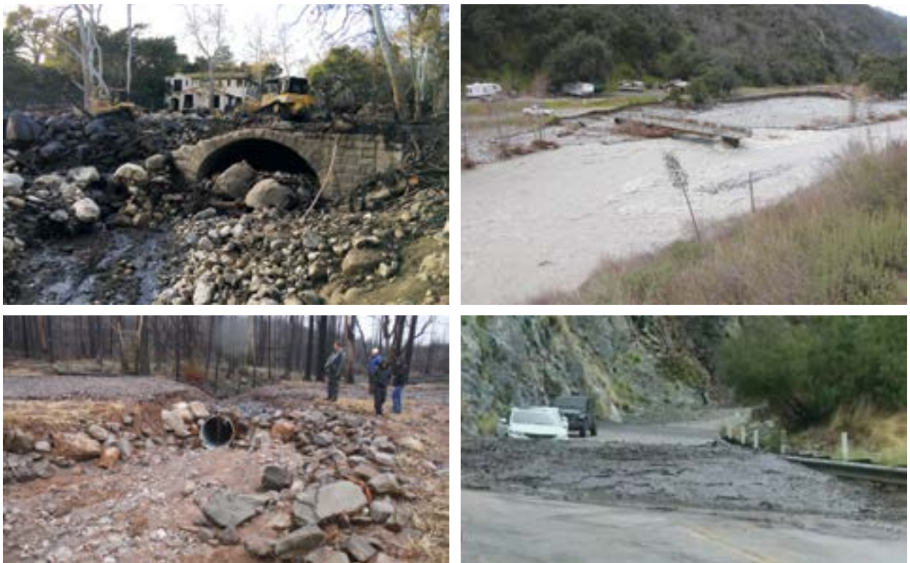
Figure 4.7—Roads, culverts, and bridges are the infrastructure most affected by geologic hazards, especially landslides, debris flows, and floods. Left photos by Donald Lindsay, upper right photo by Alan Yamada, lower right photo by Allen King.
