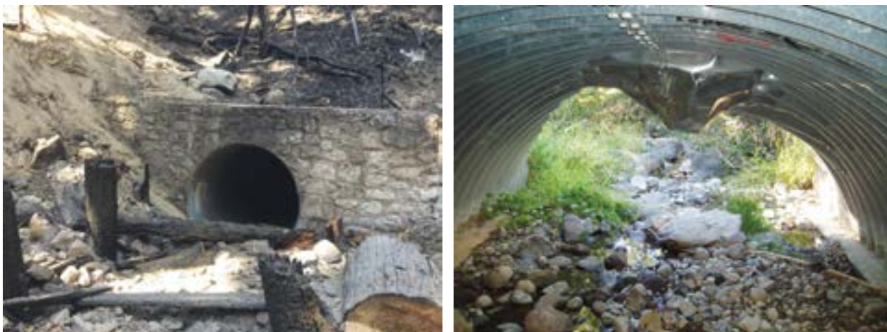
Figure 4.38—Culverts needing maintenance or repair and with a high risk of failure from plugging because of logs across the inlet and damage to the inlet. Left photo by Donald Lindsay, right photo by Gordon Keller.
