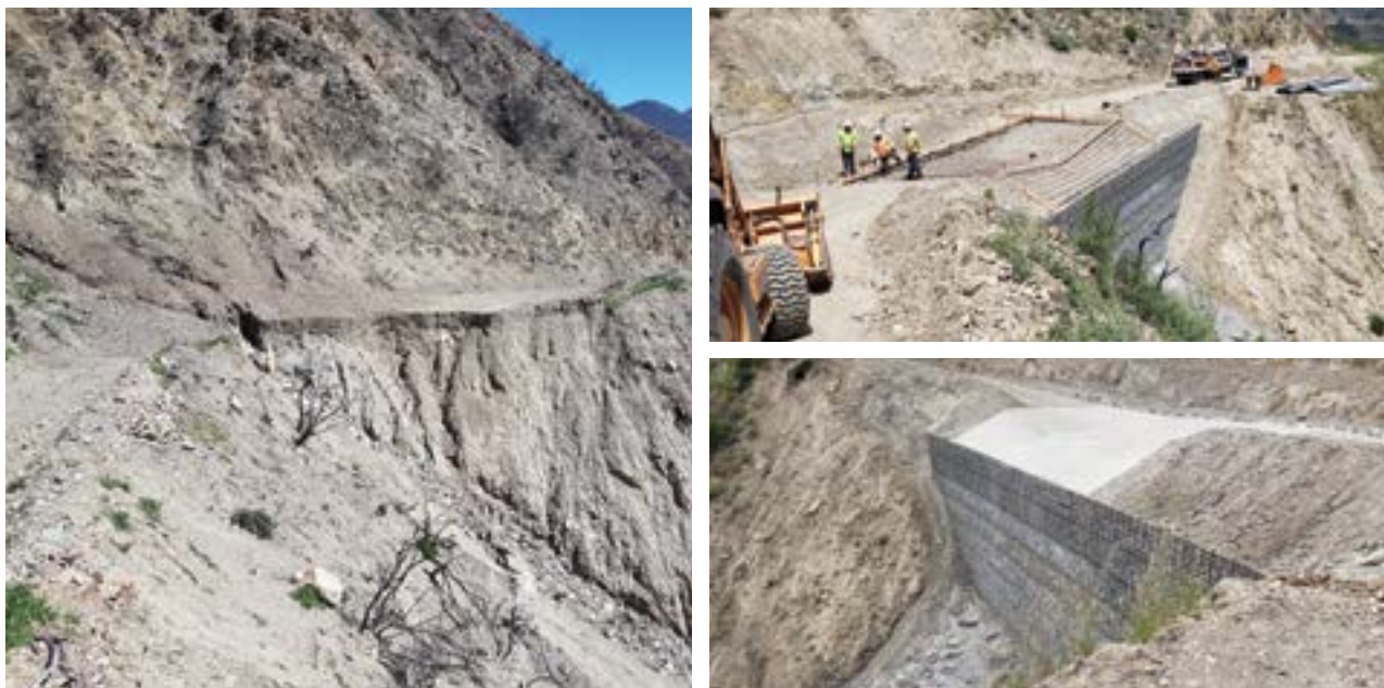
Figure 4.34—A washout on a forest road after a fire and storm event. The site was repaired with an armored dip, retaining wall, and grouted riprap below the wall. Photos by Joshua Direen, USDA Forest Service, San Bernardino National Forest.
