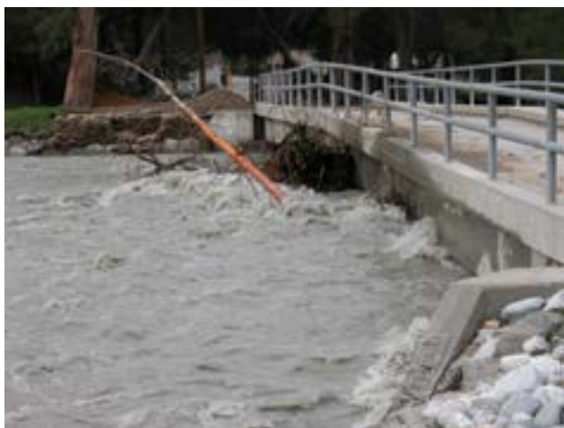
Figure 4.49—A failed bridge and road approach closed during the Angeles National Forest major 2005 storm event (top). A bridge with minimal freeboard (bottom) runs the risk of failure, particularly if a debris flow hits the bridge. Photos courtesy of Alan Yamada.
