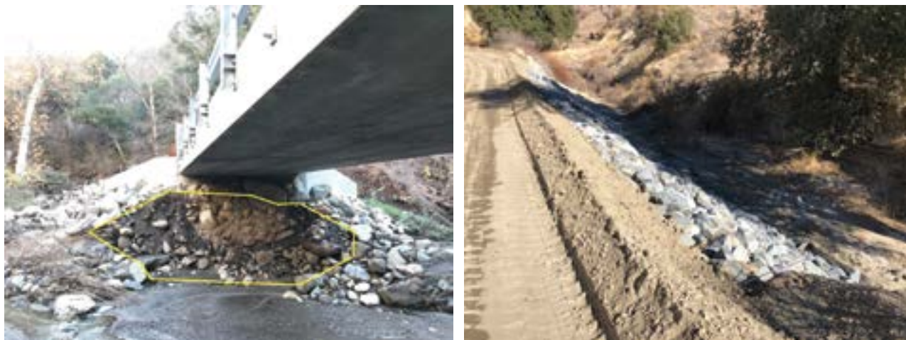
Figure 4.21—Common channel (right) and streambank (left) stabilization using rock riprap. Note where riprap has been washed away from a bridge abutment (yellow polygon) because the riprap rocks were too small. Left photo courtesy of Leslie Boak; right by Joshua Direen, USDA Forest Service, San Bernardino National Forest.
