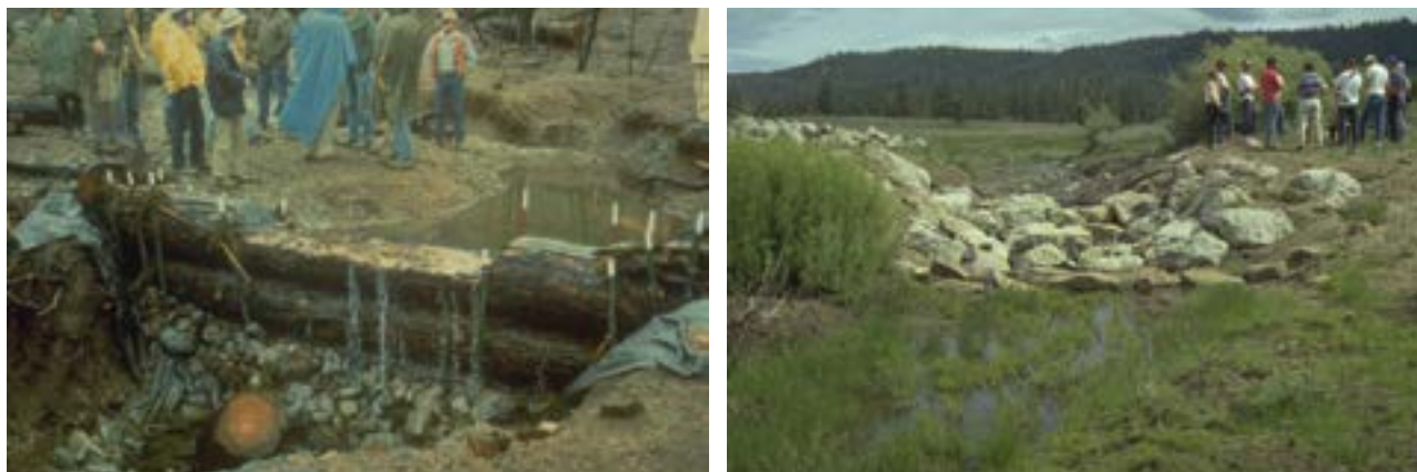
Figure 4.60—Gully stabilization structures made from logs (left) and of loose rock (right). Photos by Gordon Keller.
