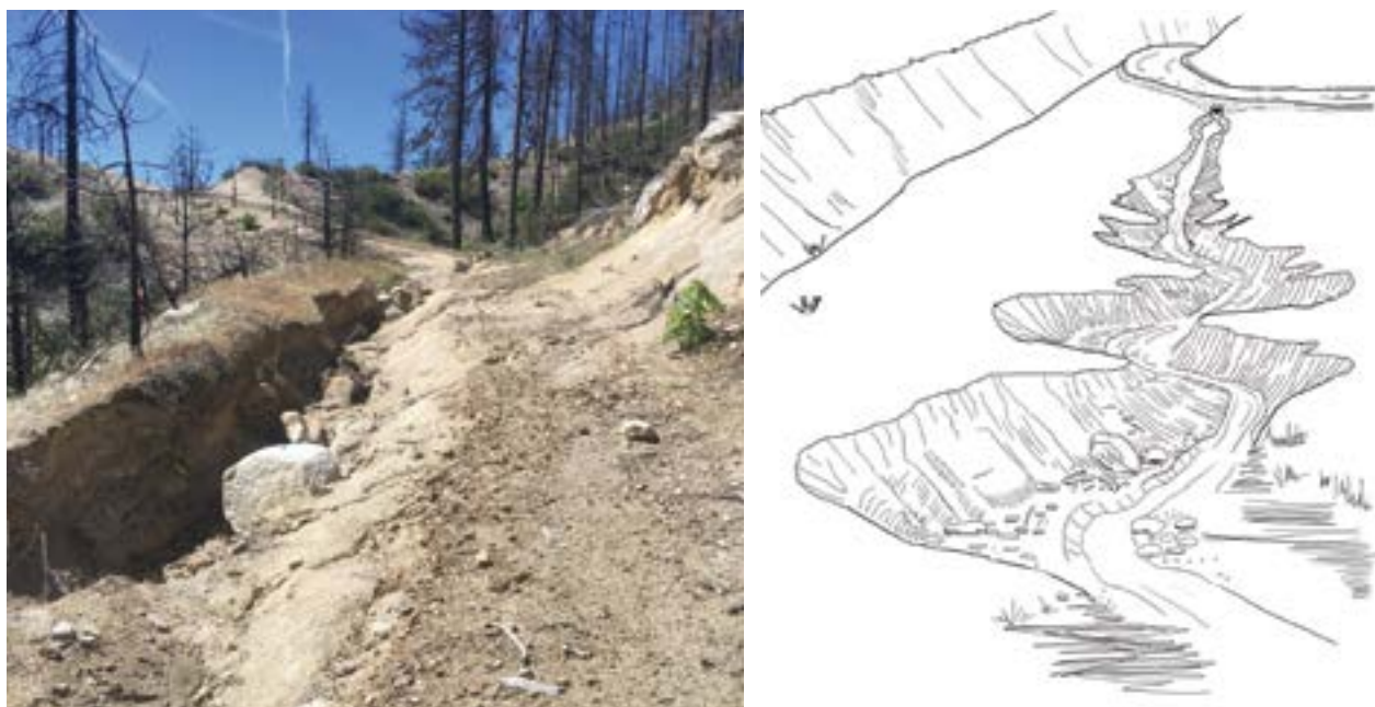
Figure 4.58—Gully formation below a road where excessive water was discharged from a ditch-relief cross-drain culvert (left) and in a ditch line below a wildfire area after a thunderstorm (right). Illustration by Heather Ross, photo by Donald Lindsay.
