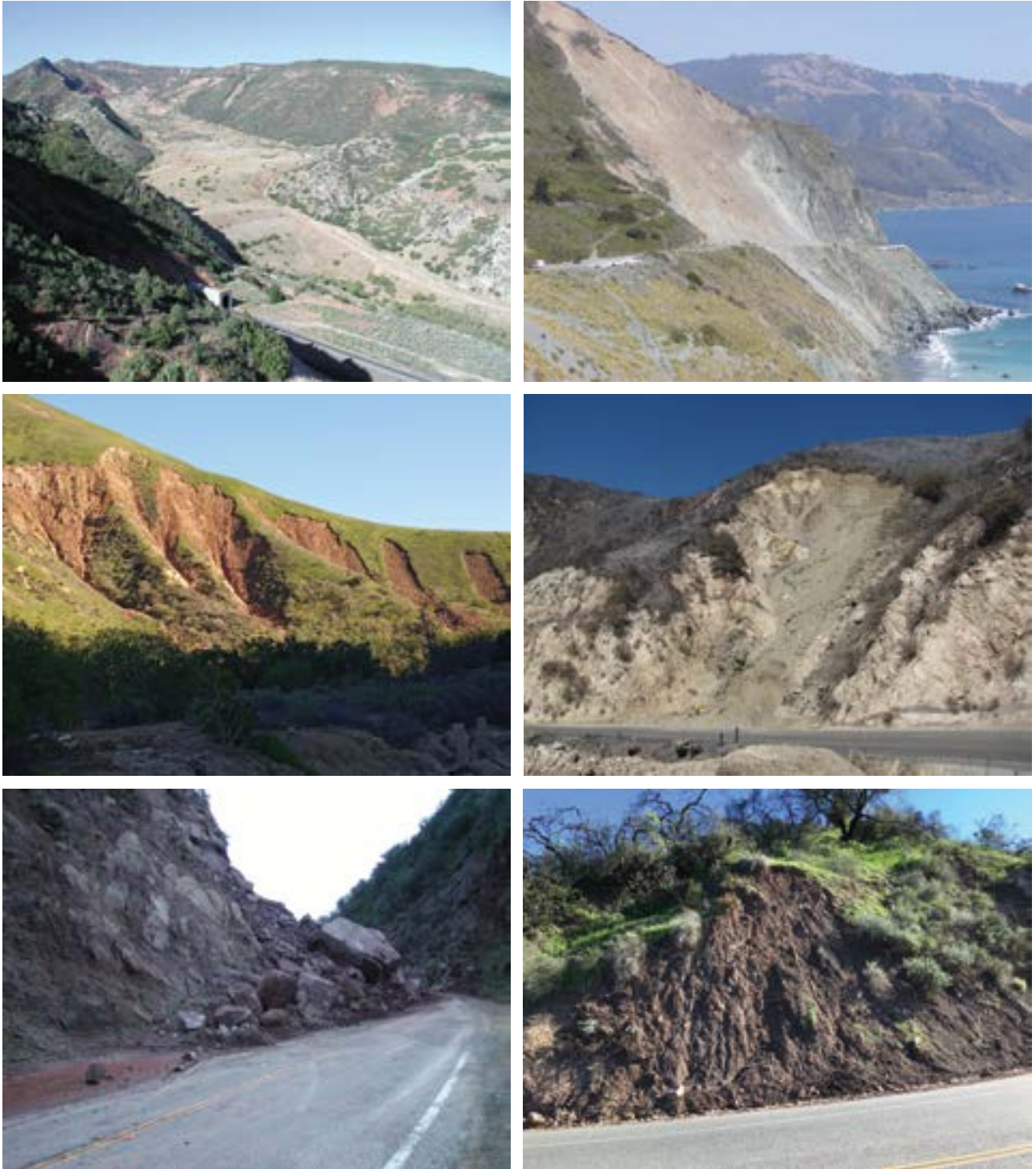
Figure 4.62—Examples of the variety of slope instability types seen on national forests in southern California, ranging from large earthflows and landslides to local rockfall and road cut slumps. Top, middle, and bottom left photos by Allen King; bottom right photo by Gordon Keller.
