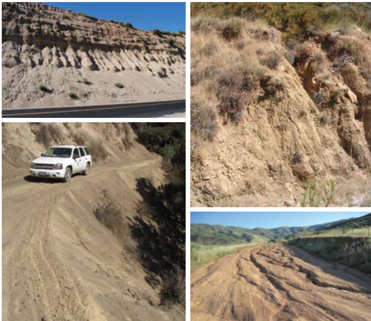
Figure 4.54—Common soil erosion problems and potential erosion along roads. Photos by Vincent Barandino, USDA Forest Service, National Technology and Development Program; except lower left photo by Allen King.
