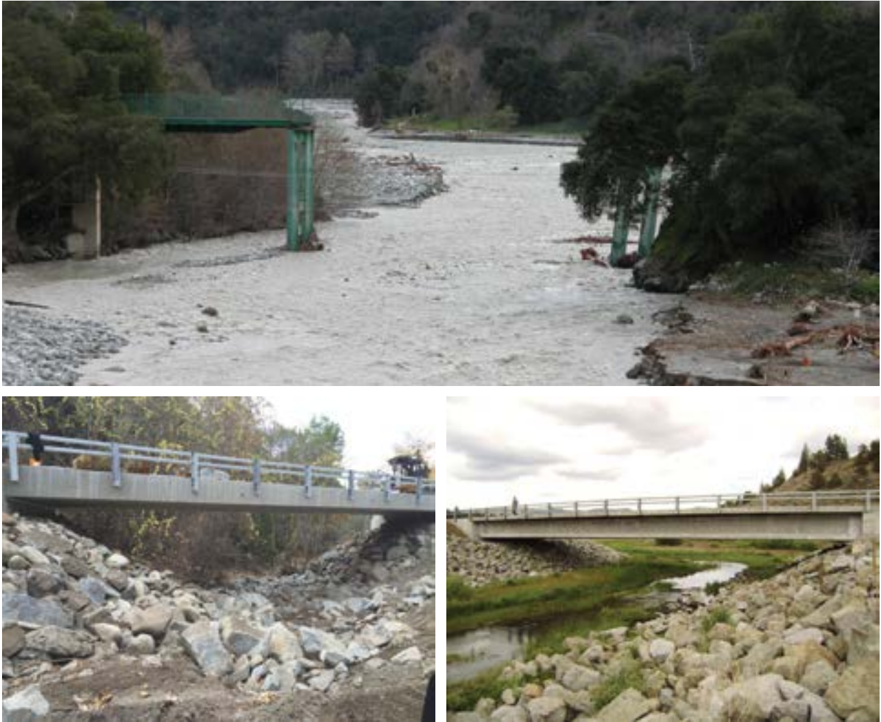
Figure 4.53—A bridge that failed as a result of scour around its right pier and abutment (note the leaning pier) (top), and bridges with scour protection provided by rock riprap around the abutments (bottom). Protection is essential for bridges that are constructed on stream bends. Upper photo by Alan Yamada, lower left photo by Kirsten Winter, lower right photo by Gordon Keller.
