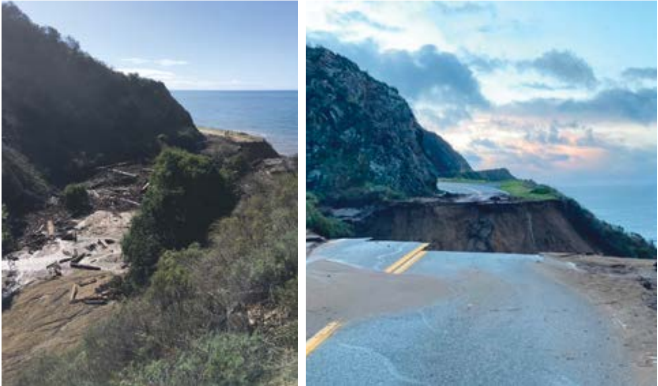
Figure 4.9—A 2021 debris flow, caused by heavy rain in the Rat Creek watershed after the 2020 Dolan Fire, plugged a major culvert and subsequently washed out a portion of California State Highway 1. The highway was closed for 3 months. Photos by Donald Lindsay.
