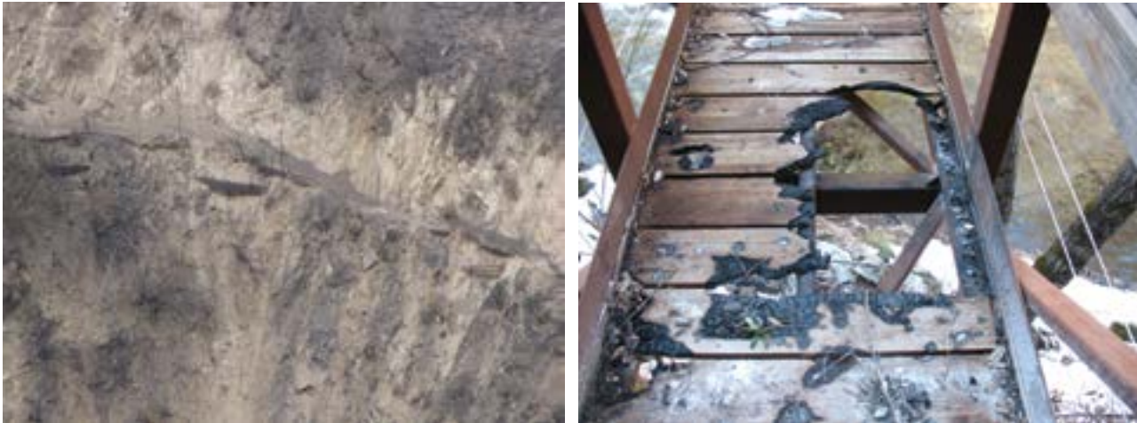
Figure 4.75—Damage to trails and trail bridges after a fire. Structures may need replacing, and sections of trail may require heavy maintenance or reconstruction. Left photo by Allen King, right photo by Jonathan Berry.
