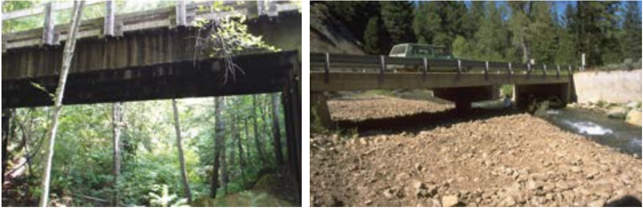
Figure 4.50—Stream channels under bridges occasionally need clearing and tree or sediment removal to maintain channel capacity and prevent blocking and diverting flows and plugging the bridge. Point bars (right) will repeatedly build up with time, creating a continual maintenance problem at bridge sites. Bends are often poor locations for bridge sites because of persistent sediment deposition and channel changes. Photos by Gordon Keller.
