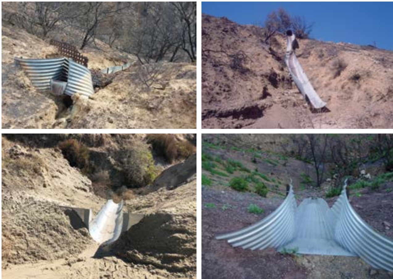
Figure 4.33—Metal flume overside drains damaged by storms and the Cottonwood and Ojai Fires (top) and new installations of downdrains (bottom). Note the critical area at the inlet that often fails without proper installation and compaction. Left photos by Joshua Direen, USDA Forest Service, San Bernardino National Forest; right photos by Gordon Keller.
