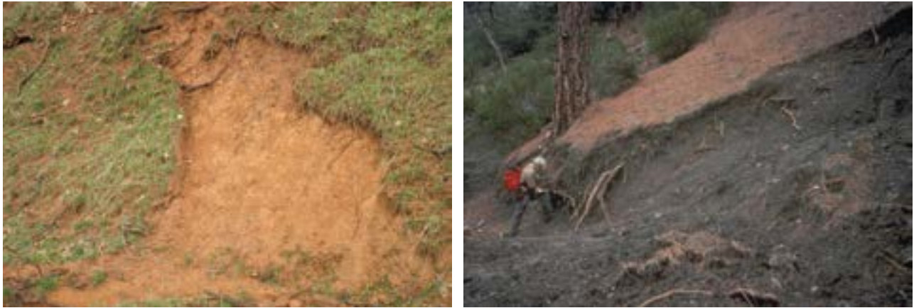
Figure 4.67—A shallow failure at the depth of shallow-rooted grasses (left) and a deep-rooted system from pine tree vegetation (soil bioengineering) that provides deeper stabilization to the slopes (right). Left photo by Gordon Keller, right photo by Donald Gray.
