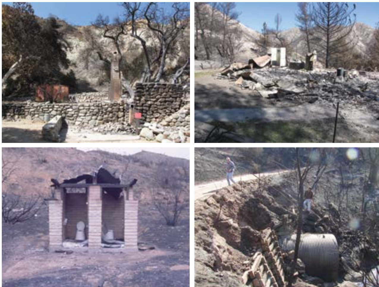
Figure 4.2—Forest infrastructure. Wildfires often damage administrative sites, recreation facilities, and other infrastructure (including walls, culverts, and bridges) such as these. Upper photos by Allen King, and lower photos by Gordon Keller.
