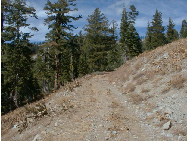
Figure 2a. Typical low use road in the Tahoe Basin. Note the existing ruts, negating the benefits of outsloping (Villanueva, 2013).
